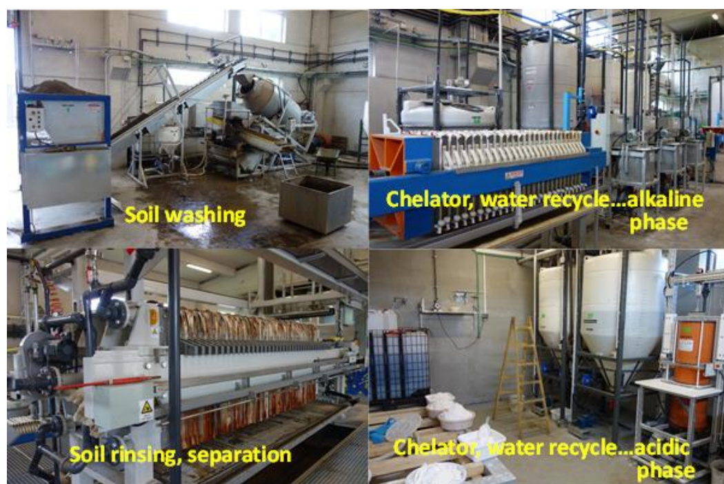
Figure 1: Demonstrational soil-washing plant (TRL 7) with ReSoil technology in the city of Prevalje, Slovenia. The plant with capacity of 1.5 tons of soil per batch is operated by Envit Ltd. The plant construction was supported by the EU project LIFE12 ENV/SI/000969 ( http://www.envit.si/ ).
