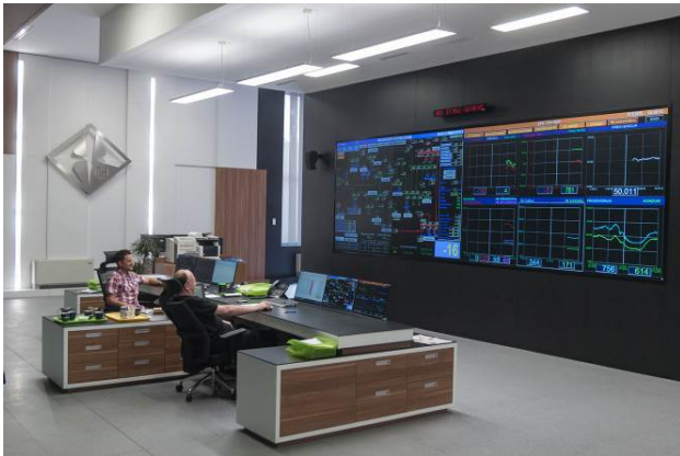
Figure 5: Command and control centers (JPEP BiH - NC)
