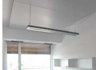
Figure 5. Heating/cooling ceiling panels in refurbished offices.
