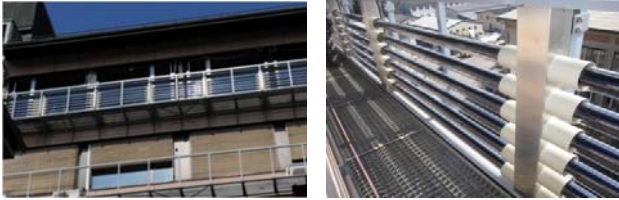
Figure 3. Air-heating vacuum tube collectors on the pilot site.
